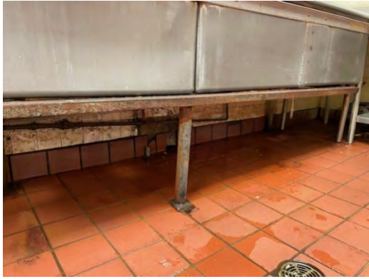
Rusted Kitchen Equipment
