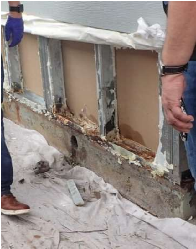
Rusted sill tracks
