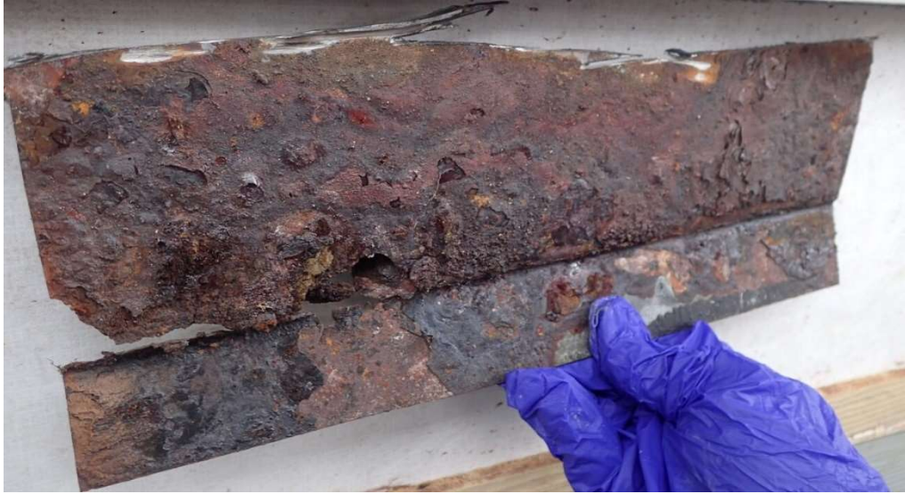
Corroding sill track
