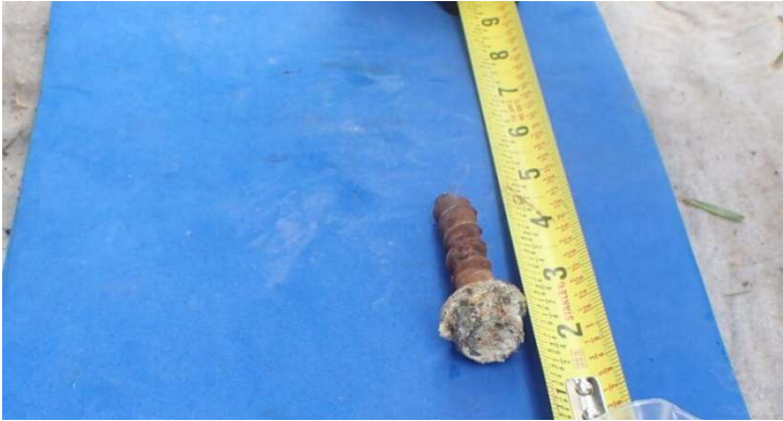
Rusted anchor screw that snapped off
