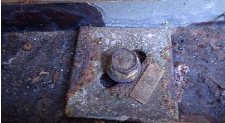
Rusted sill track and anchor screw
