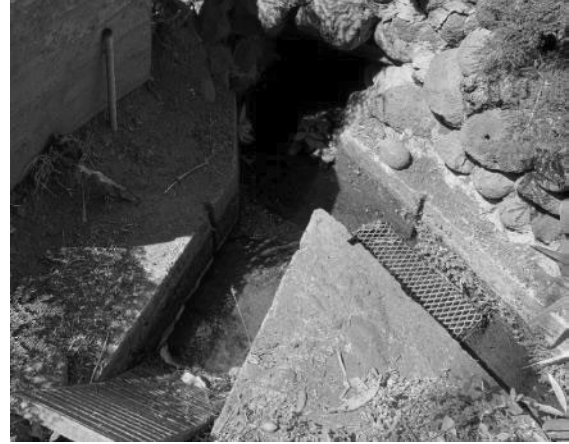
D) Water flows from a driveway culvert at the Velez property and towards Velez, Ciotti, and Ibara.
