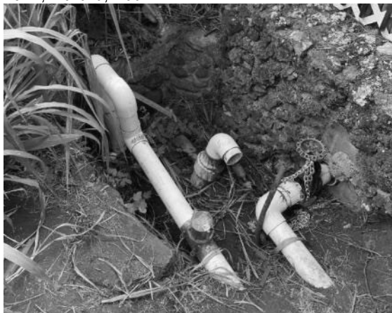
A) Distribution pipe with valve chained and flow meter at center, located on the boundary of Imua Family Services property.
