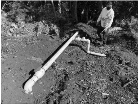
C) Newly installed lateral 4-inch line from Waikapu Properties’ line continues to South Waikapū Kuleana ‘Auwai.
