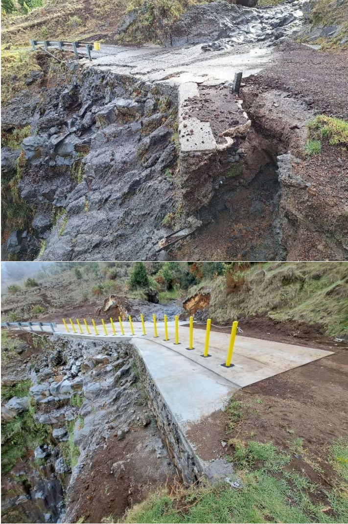
Figure 3. Storm damage to a cement stream crossing on Waipoli Road in the KFR and the same crossing after repairs.
