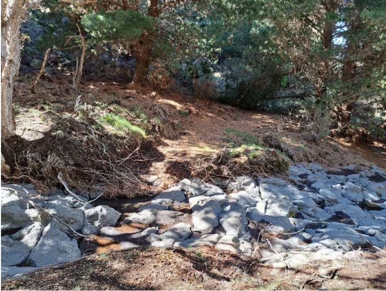
Figure 5. Kona Low Storm damage to stream crossing spillway #6.
