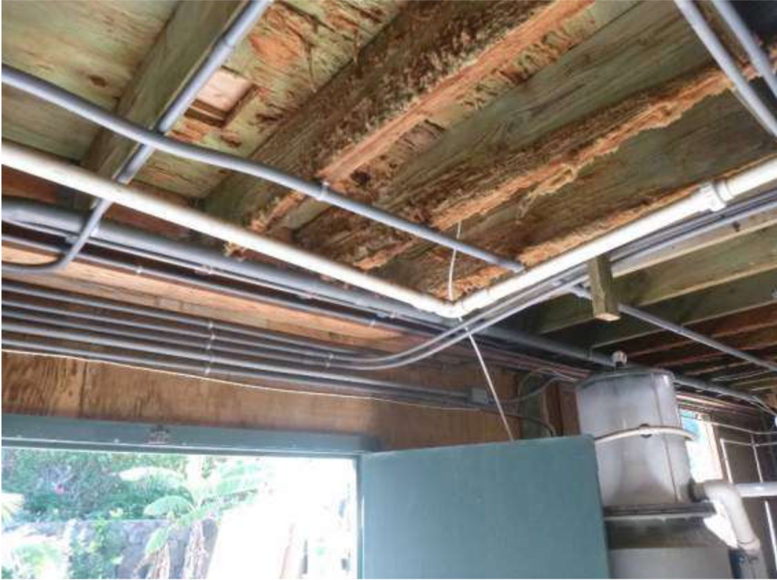
Fig. 2. Damaged joists and plywood under OI's fish and shrimp hatchery.
