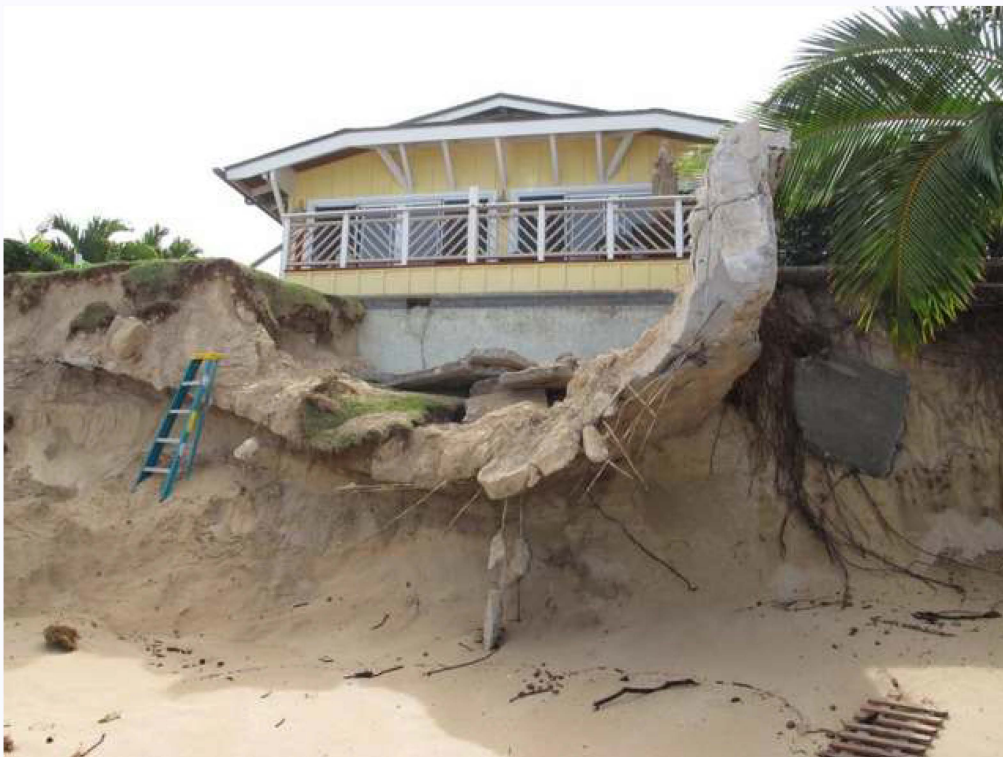
House threatened by erosion on North Shore of O'ahu.
