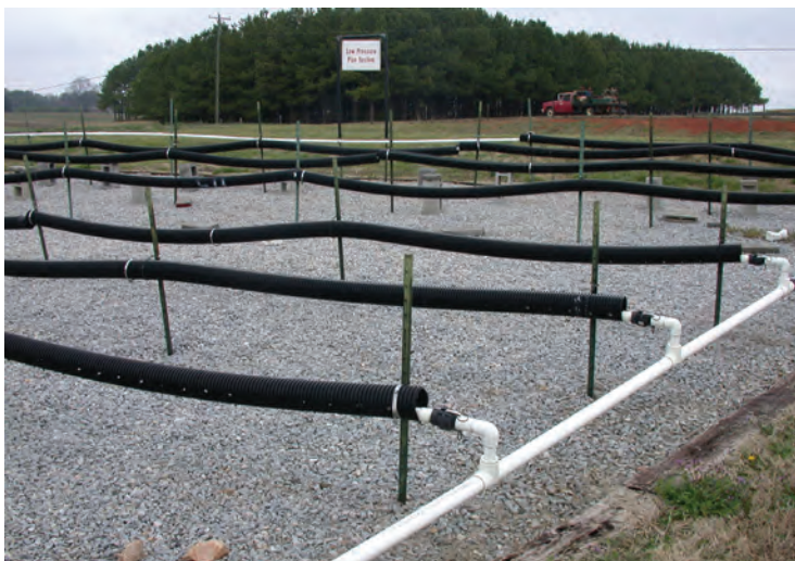
Low Pressure Pipe Disposal System Demonstration (North Carolina State University).
