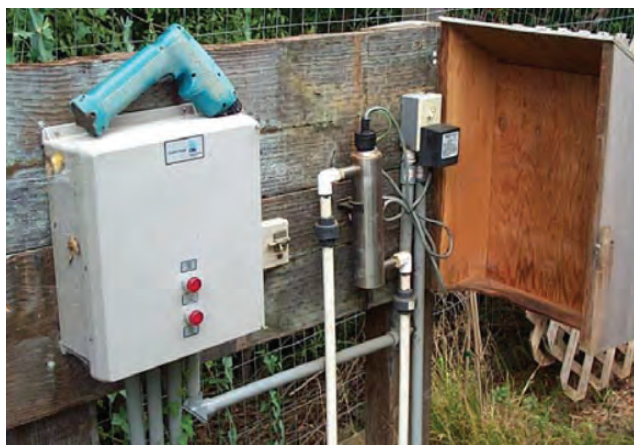
An ultraviolet disinfection system (steel cylinder to the right of the control box) used to treat sand filter effluent before landscape irrigation.
