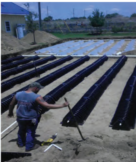
Gravelless Absorption Bed Disposal System.
