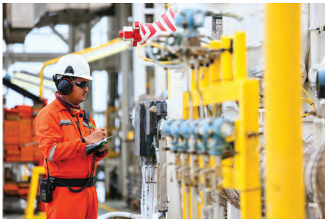
FIGURE 9. System Testing Decentralized wastewater systems would be subject to the same operator licensing, rules, and requirements current in place for existing wastewater treatment plants.
