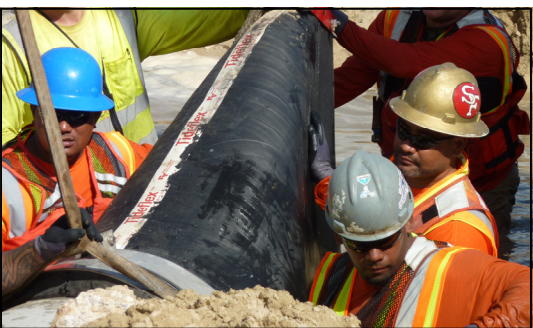
The City & County workers work hard to remove the "duck bill." The surrounding sand forced it to close causing Pokiwai stream to become stagnant.
