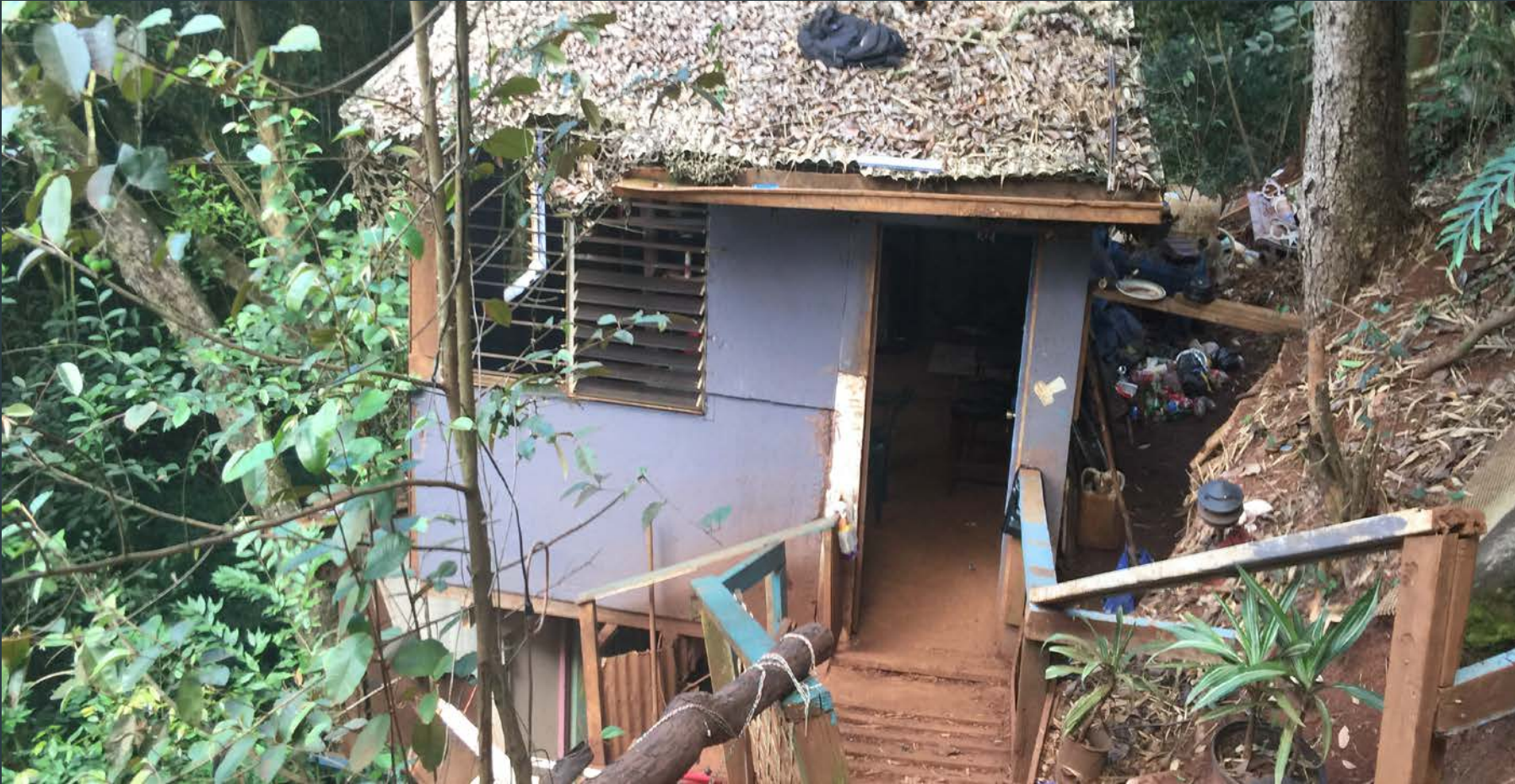
Photo of unpermitted structure behind the Whitmore Circle Apartments.
