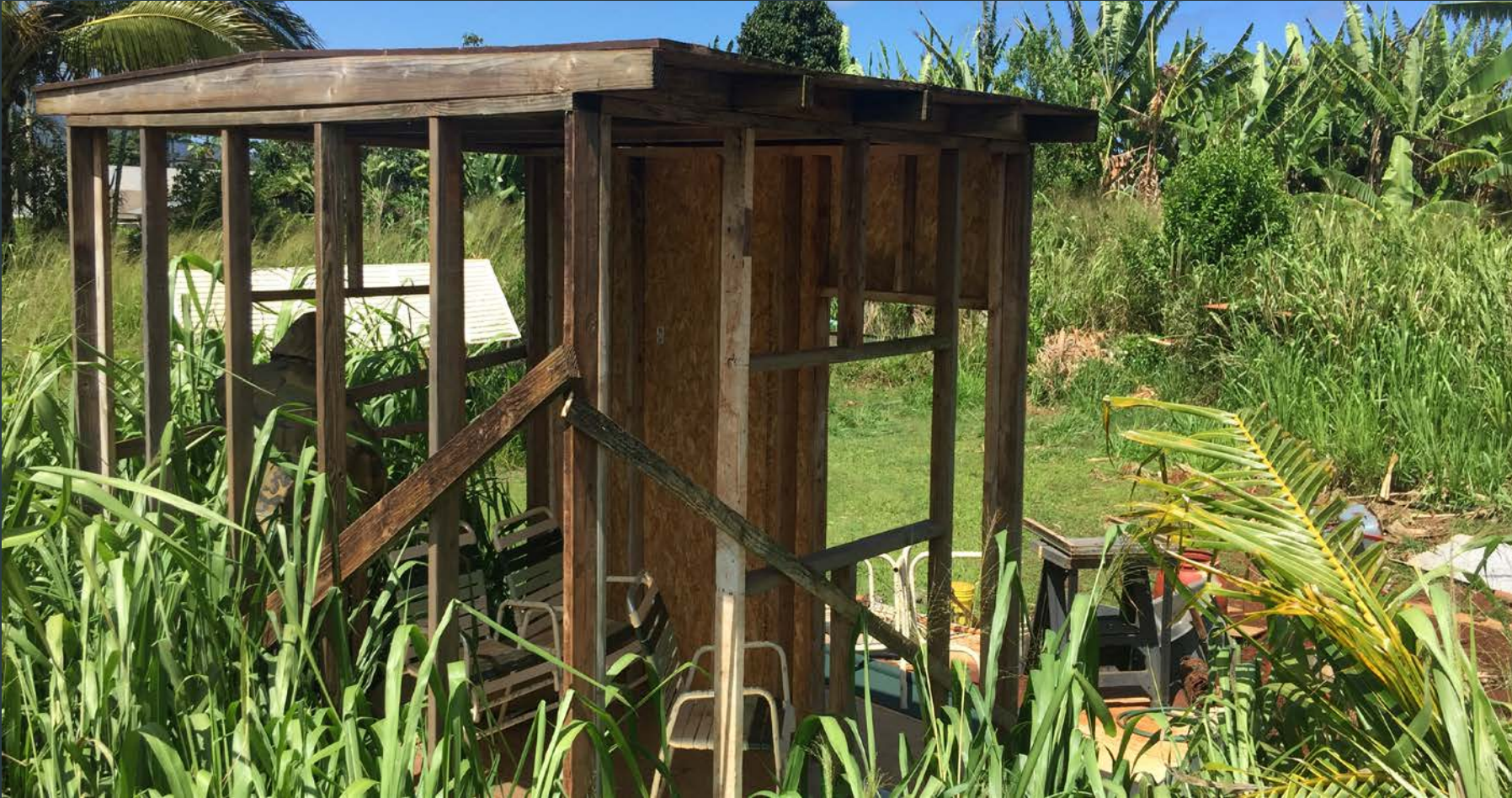
Unpermitted structure located on State property.
