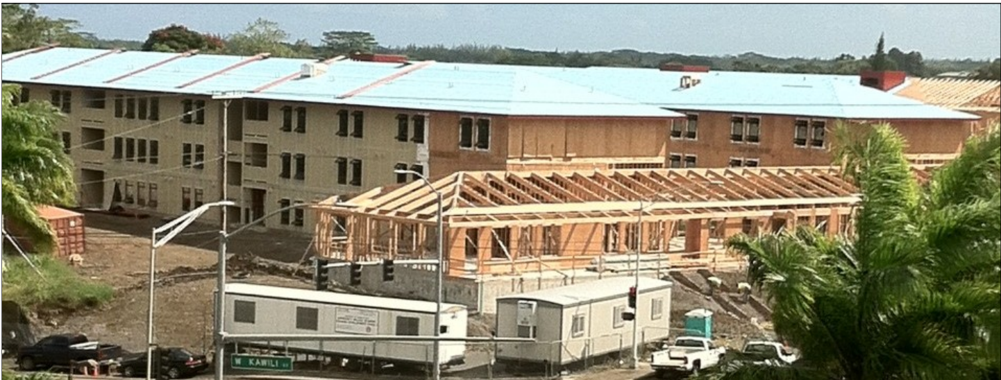
The new University Village Phase I at University of Hawaii at Hilo is the result of a $32 million appropriation by the Legislature in 2011 and will include approximately 300 student housing units in apartments and suite style rooms opening this summer.
