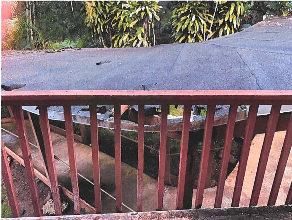
Photos 2 & 3 – Covered Walkway Roof – broken with holes in multiple areas.
