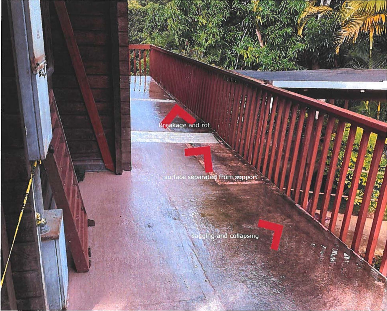
Photo 6: Lanai – Structurally unsound and unusable.
