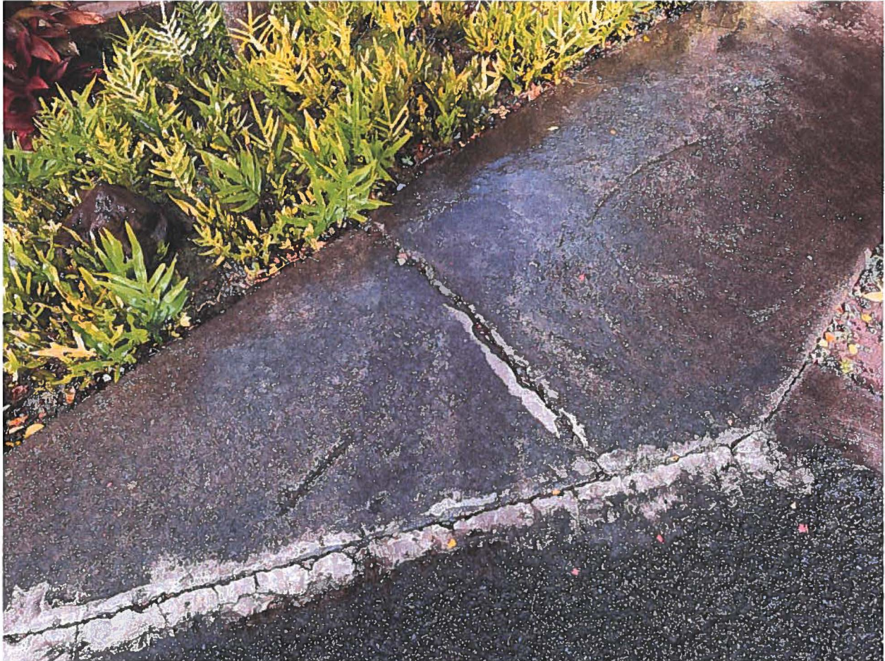
Photo 10: Parking lot – numerous cracks, pits and broken present tripping hazards for seniors.
