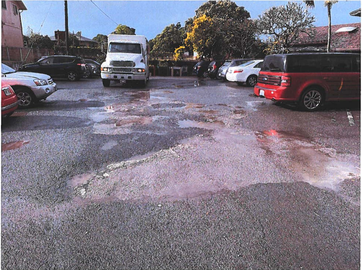
Photo 9: Parking Lot – water pools in pitted areas throughout the lot.
