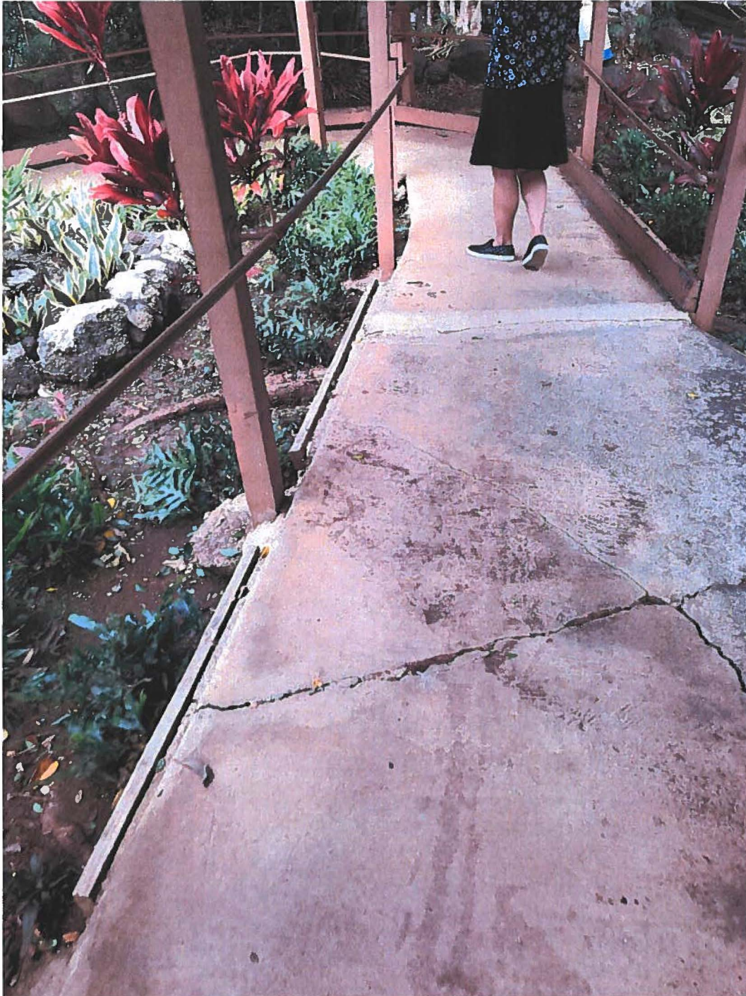
Photo 4: Walkway – Cracks and uneven surfaces throughout walkway present tripping hazards.
