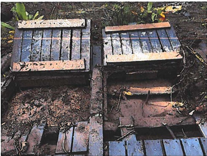
Septic System Filled w/ Mud and Debris
