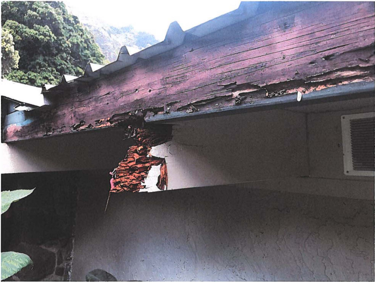
Maui Primary Programmatic Building – Rotten Rafters & Fascia
