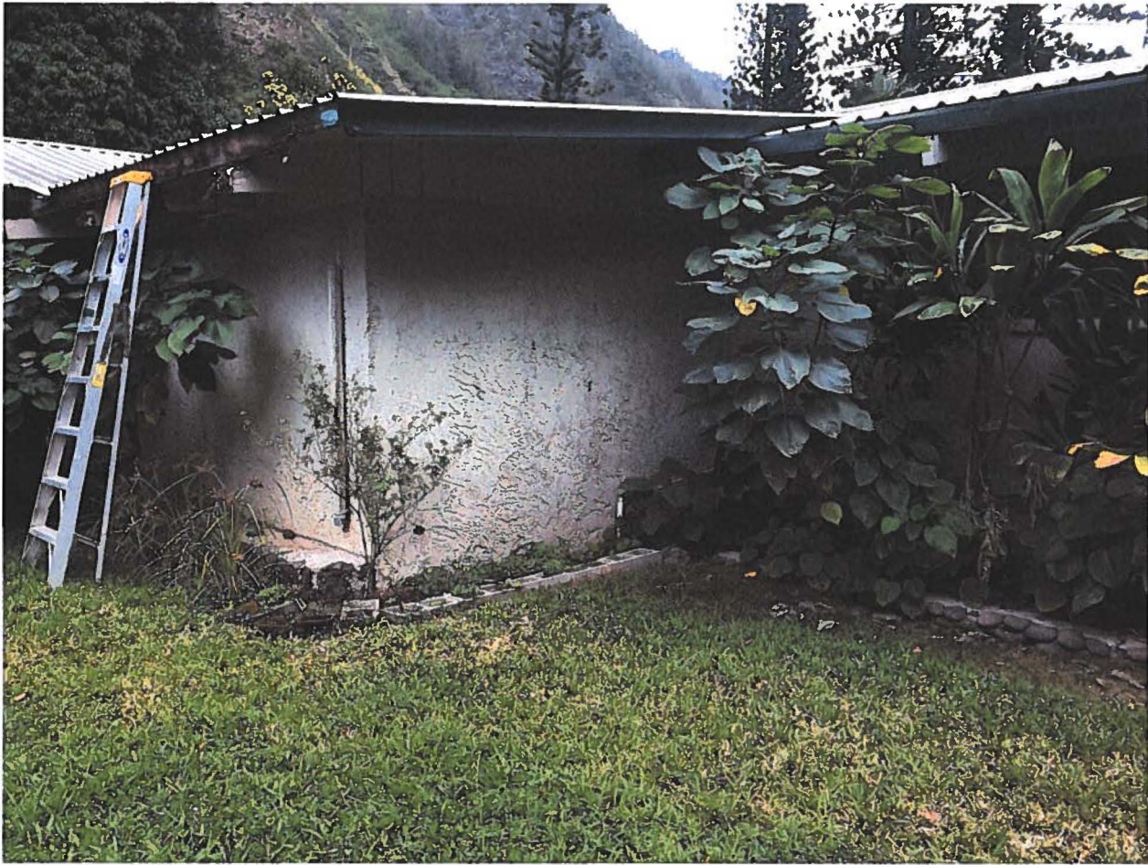
Maui Primary Programmatic Building – Whole Back Side Showing Rotten Rafters, Fascia, and Gutters
