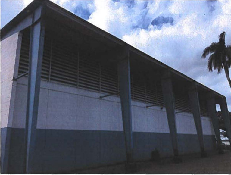
Exterior photo of gym needing Renovation.
