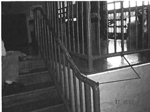
Sample no: 305-P15. Game Room to Lounge Area. Blue w/ light yellow underlayer metal handrail (same as guardrail on lounge floor).
