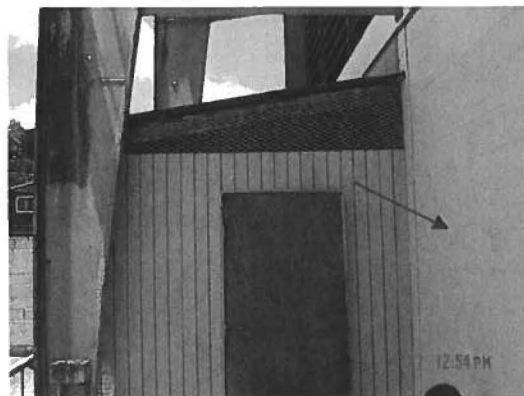
Sample no: 305-P21. Gymnasium. Light blue concrete exterior wall (swimming pool side). LCP
