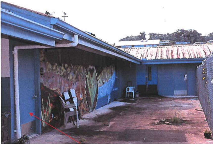
Entrance to Locker-Room Facilities, Currently Not Accessible for Physically Disabled Individuals.
