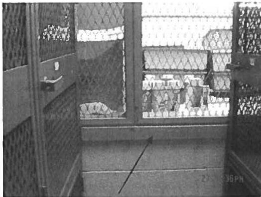
Sample no: 305-P20. Shower-Locker Room. Green wood window sill in equipment cage storage area. LCP
