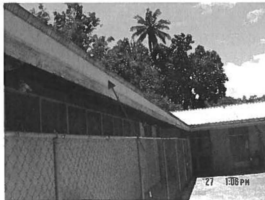
Sample no: 305-P27. Shower-Locker Room. Faded yellow metal flashing along roof. LCP
