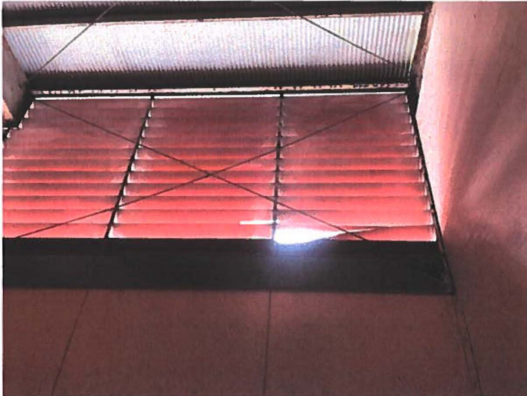
Gym slats needing repair.
