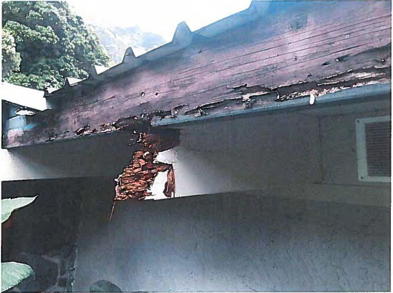
Maui Primary Programmatic Building – Rotten Rafters & Fascia
