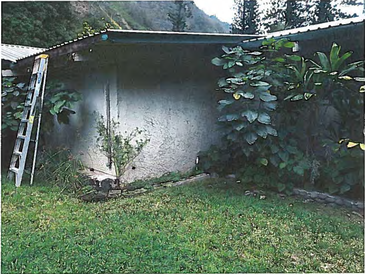
Maui Primary Programmatic Building – Whole Back Side Showing Rotten Rafters, Fascia, and Gutters
