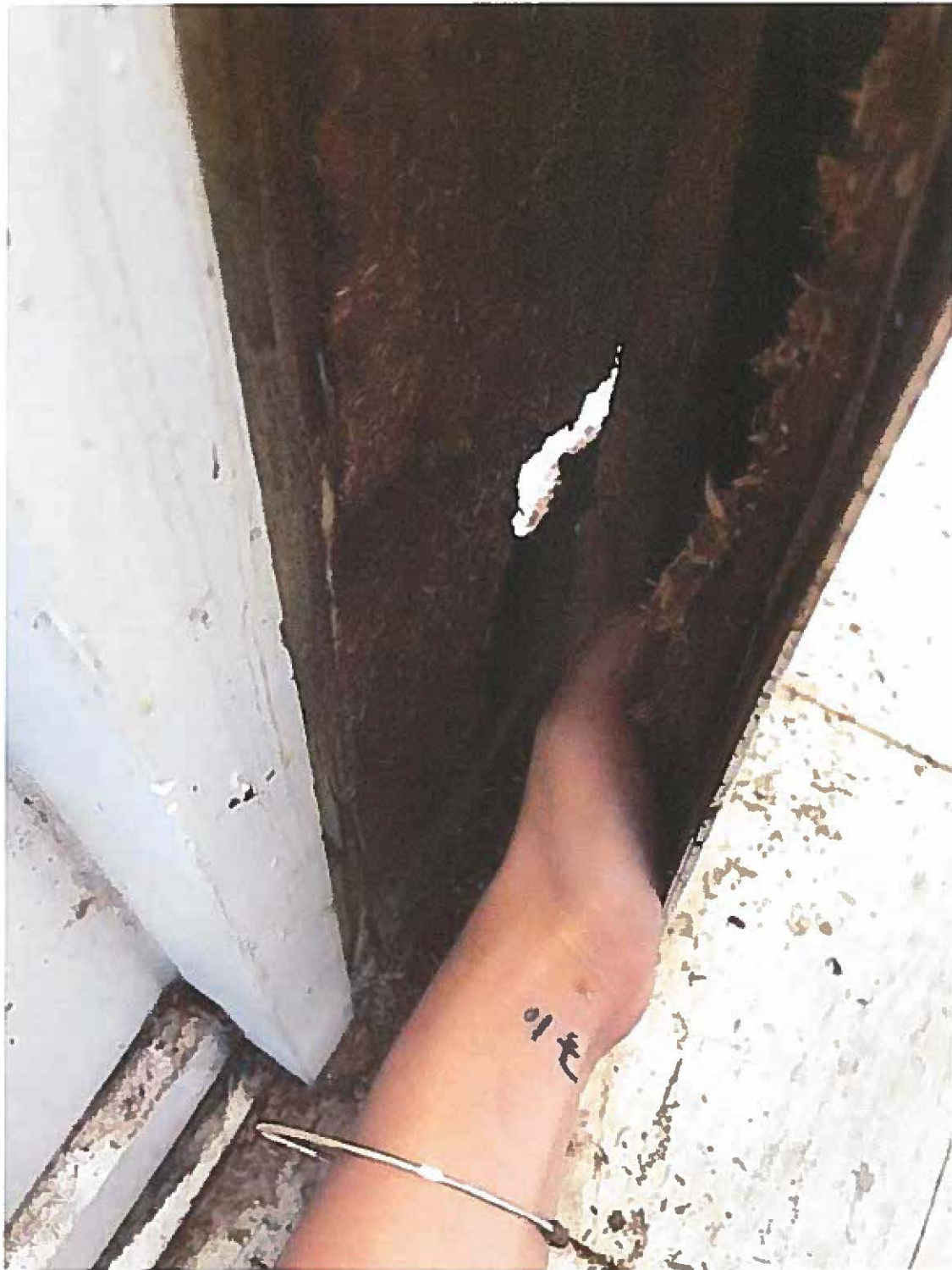
O'ahu Ranger Cottage – Crumbling Exterior Wall
