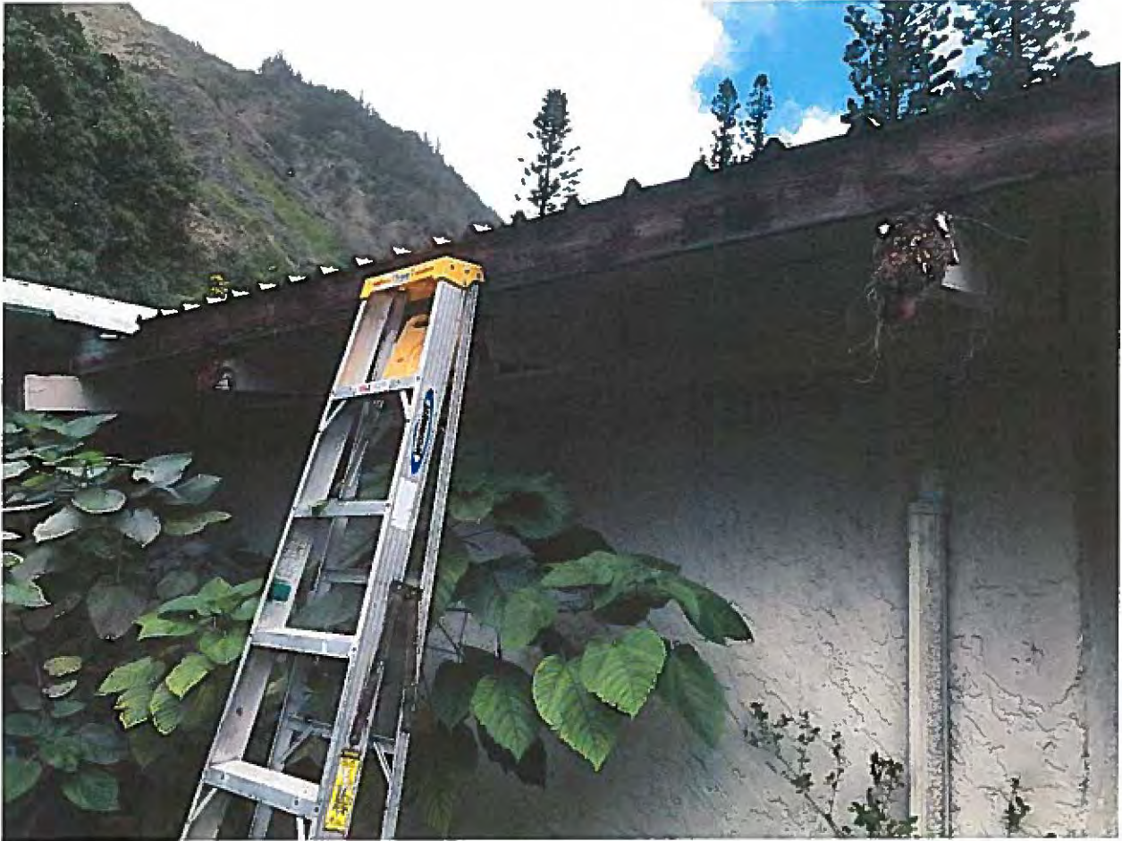
Maui Primary Programmatic Building – Rotten Rafters
