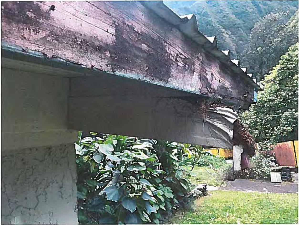
Maui Primary Programmatic Building – Rotten Rafters & Gutters
