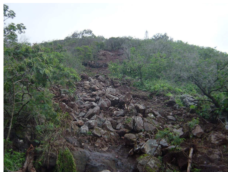
Removal of large boulders from Moanalua Valley hillsides & installation of landslide-prevention netting
